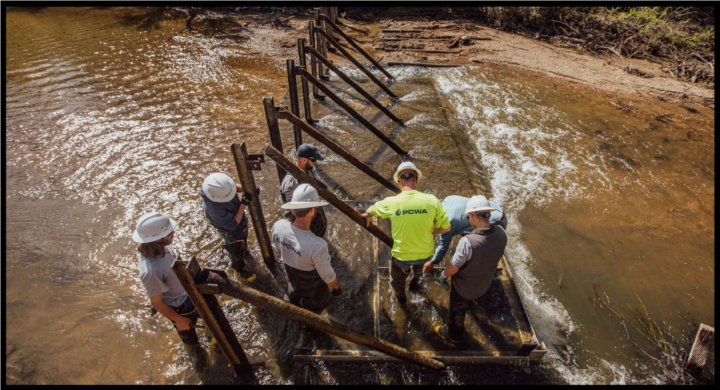
Seasonal Dam Installation, Lincoln
